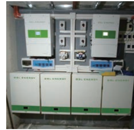
-Philippines 20kWh Hybrid Solar Storage System
