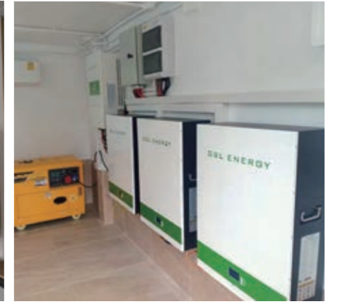
-Thailand 40kWh Hybrid Solar Storage System
