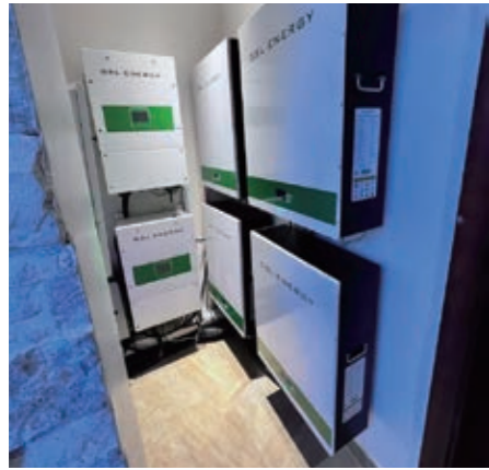
-Nigeria 40kWh Hybrid Solar Storage System
