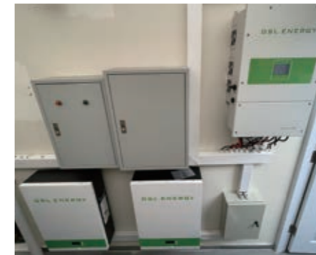
-Philippines 10kWh Hybrid Solar Storage System
