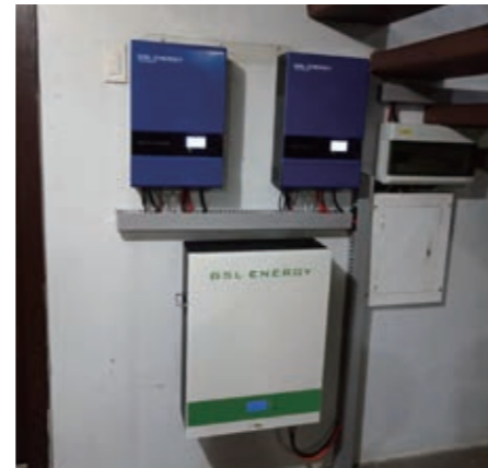
-Kenya 10kWh Hybrid Solar Storage System
