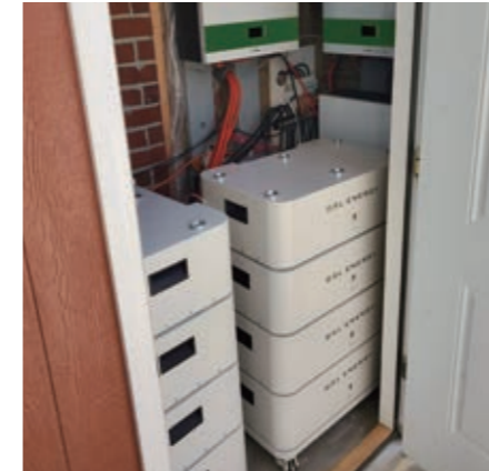
-Jamaica 40kWh Hybrid Solar Storage System
