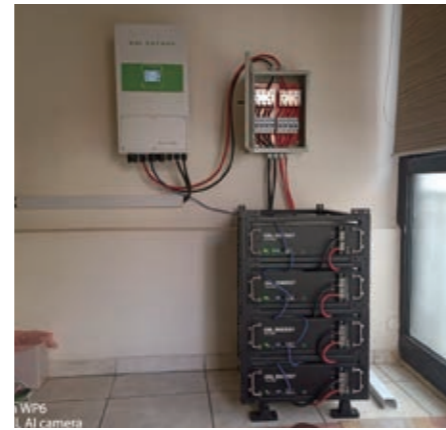
-Lebanon 20kWh Hybrid Solar Storage System
