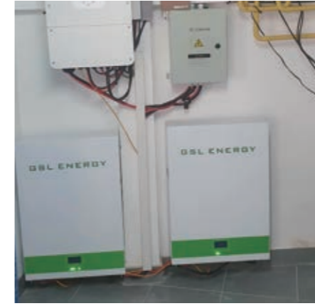
-Thailand 100kWh Hybrid Solar Storage System
