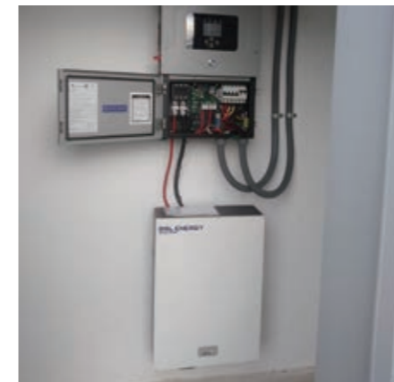
-Puerto Rico 10kWh Hybrid Solar Storage System
