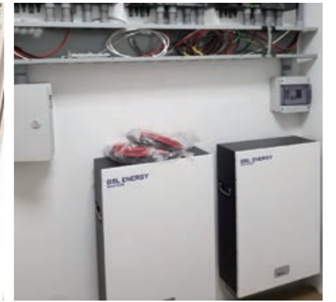
-Philippines 14.34kWh Hybrid Solar Storage System
