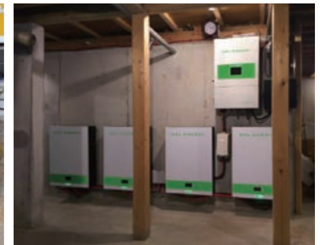
-Japan 40kWh Hybrid Solar Storage System
