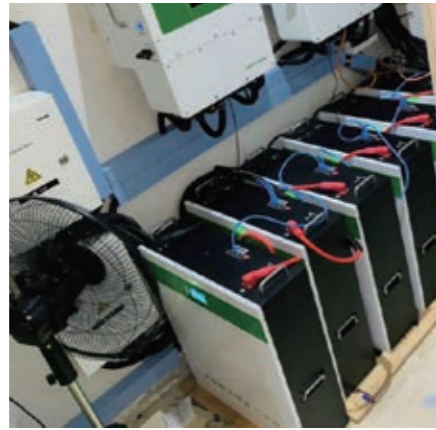
-Nigeria 60kWh Hybrid Solar Storage System
