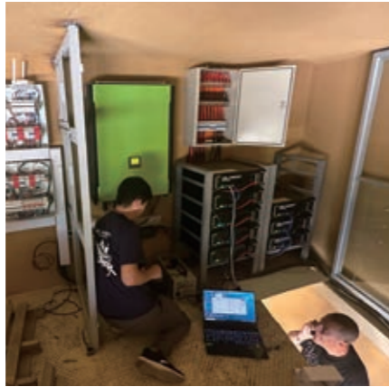
-Lebanon 40kWh Hybrid Solar Storage System
