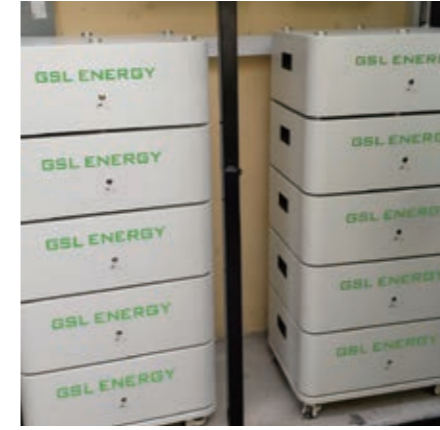
-Jamaica 100kWh Hybrid Solar Storage System
