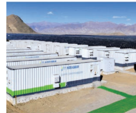
-Tibet, China 5MWh Hybrid Solar Storage System
