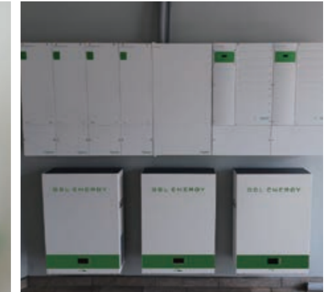
-Puerto Rico 30kWh Hybrid Solar Storage System
