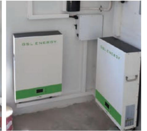
-Malaysia 20kWh Hybrid Solar Storage System
