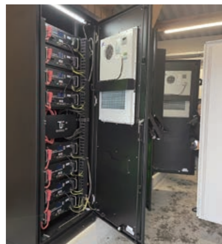
-Switzerland HV 320kWh Solar Energy System
