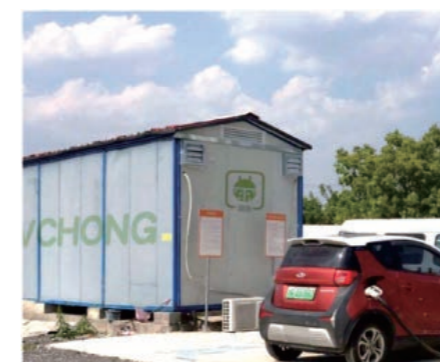
-Africa Hybrid Solar Storage System
