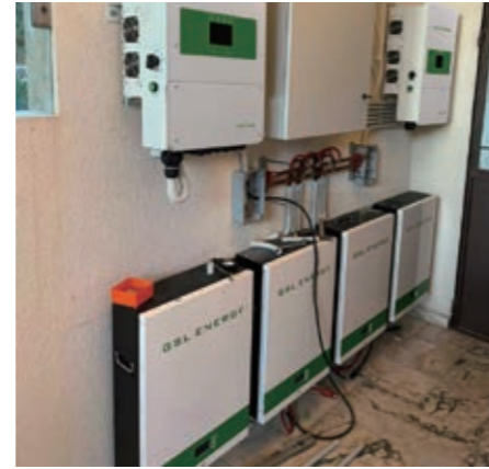
-Lebanon 20kWh Hybrid Solar Storage System
