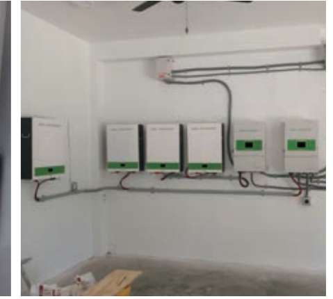
-Jamaica 40kWh Hybrid Solar Storage System
