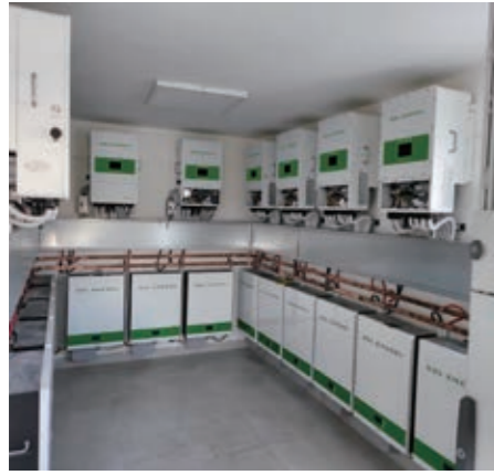
-Lebanon 140kWh Hybrid Solar Storage System
