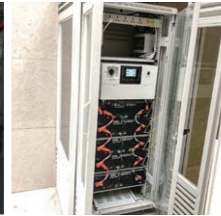
-Philippines 25kWh Hybrid Solar Storage System
