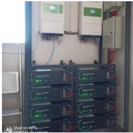
-Lebanon 40kWh Hybrid Solar Storage System
