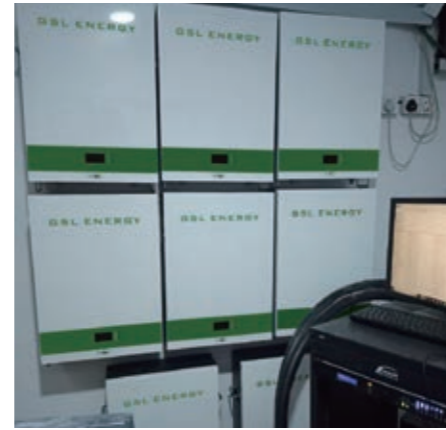
-Nigeria 80kWh Hybrid Solar Storage System
