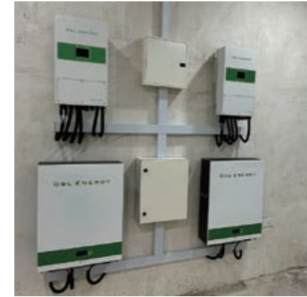
-Malaysia 20kWh Hybrid Solar Storage System
