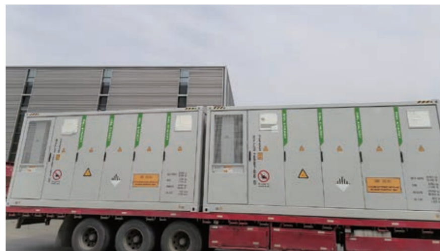
-USA 3.72MWh Liquid Cooling BESS
