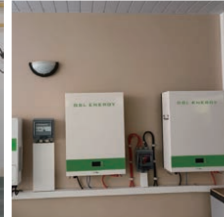
-Thailand 20kWh Hybrid Solar Storage System
