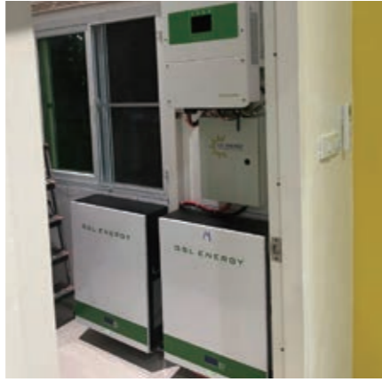
-Lebanon 20kWh Hybrid Solar Storage System
