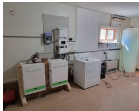
-Lebanon 40kWh Hybrid Solar Storage System
