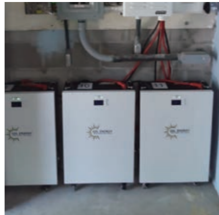
-Kenya 30kWh Hybrid Solar Storage System
