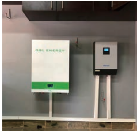
-Kenya 5kWh Hybrid Solar Storage System
