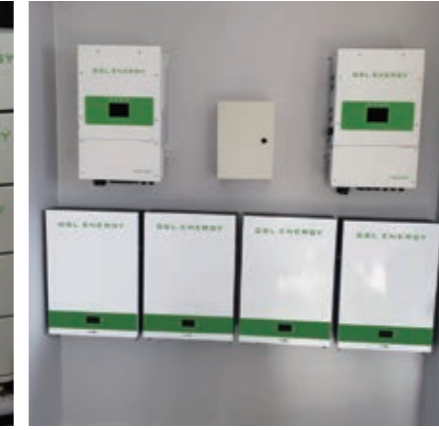
-Jamaica 20kWh Hybrid Solar Storage System
