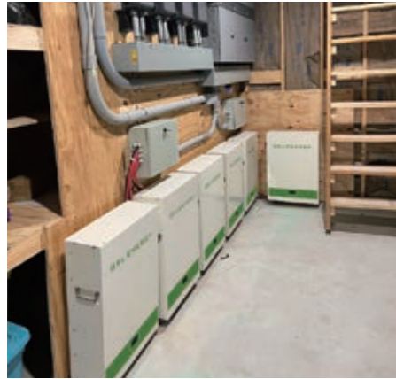
-Lebanon 60kWh Hybrid Solar Storage System
