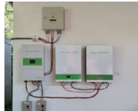
-Thailand 20kWh Hybrid Solar Storage System
