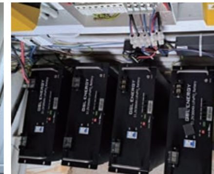
-Philippines 20kWh Hybrid Solar Storage System
