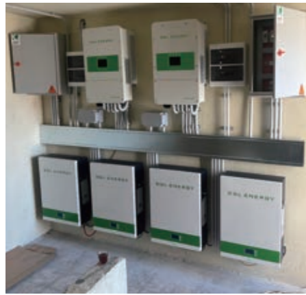
-Lebanon 40kWh Hybrid Solar Storage System
