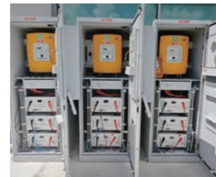
-Puerto Rico 143.4kWh Hybrid Solar Storage System
