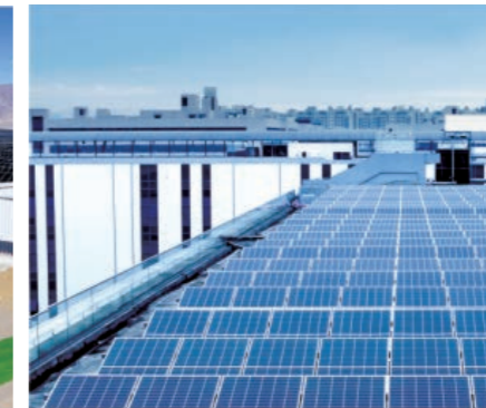
-Zhejiang, China 3MWh Hybrid Solar Storage System
