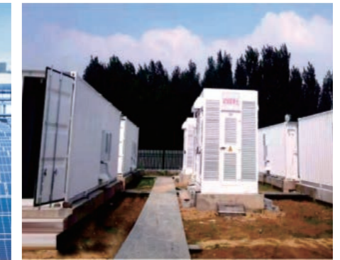
-Shandong, China 10MWh Hybrid Solar Storage System
