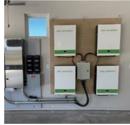
-Lebanon 40kWh Hybrid Solar Storage System
