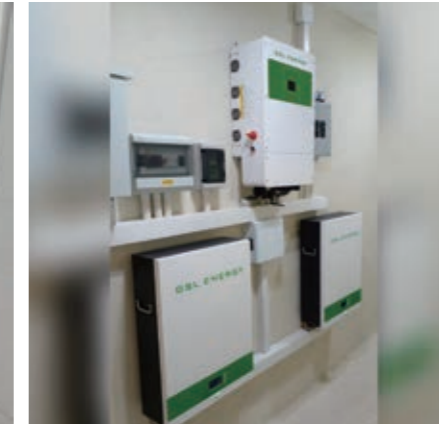
-Jamaica 20kWh Hybrid Solar Storage System
