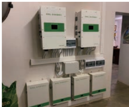
-Thailand 40kWh Hybrid Solar Storage System
